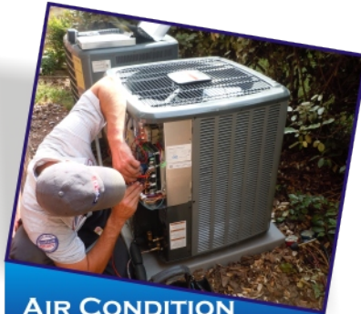
AIR CONDITION MECHANIC
